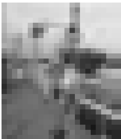
Close-up of end of loading arm fittings, showing valving that allows purging prior to disconnecting, threaded fitting for connection to tank car valve and bonding wire around loading arm swivel joints.
